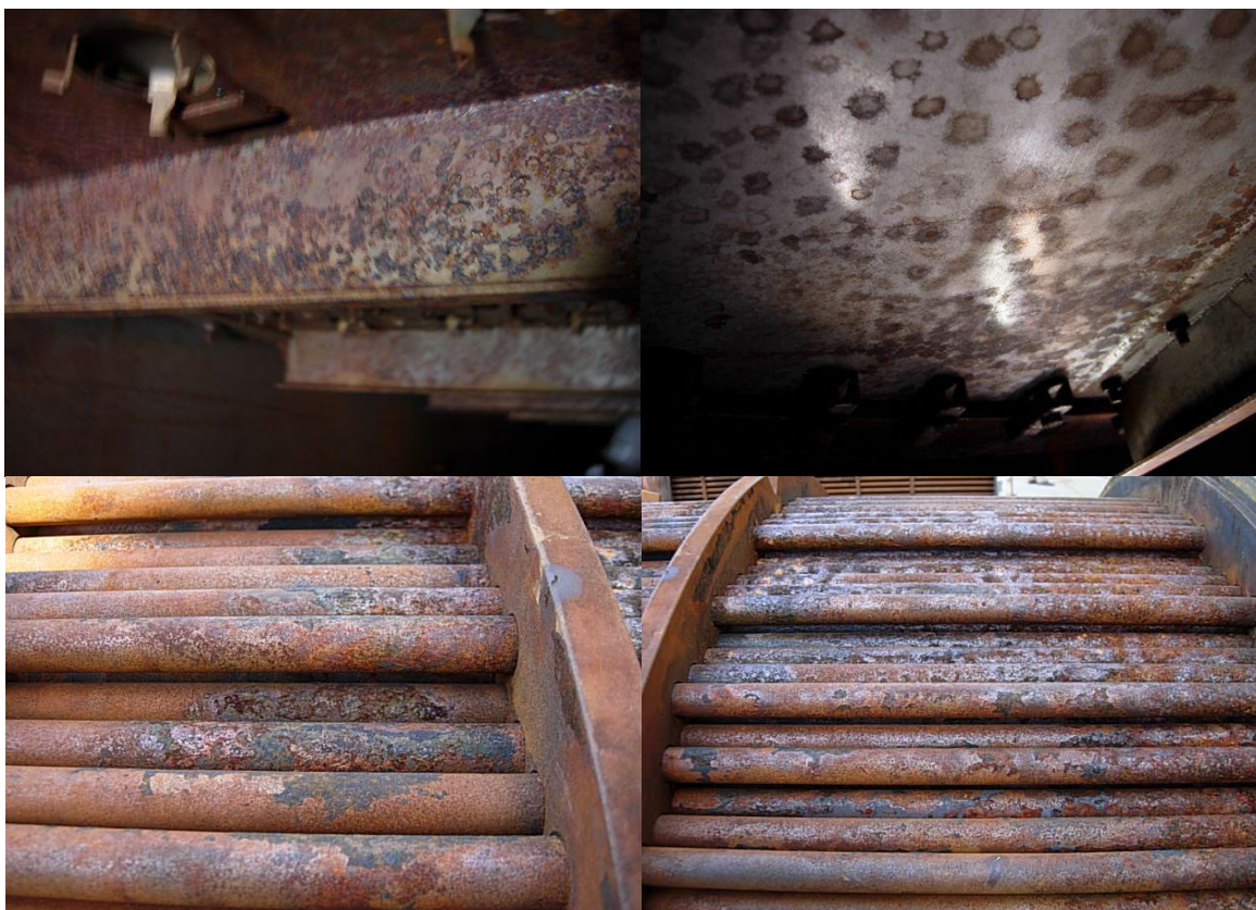
Figure 1. Photographs show the corrosion damages on different plant locations.
