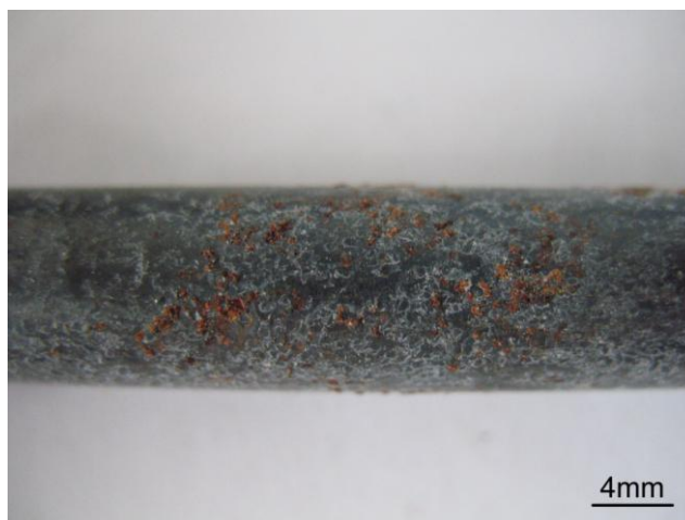
Figure 5. Corrosion morphology of the rebar after curing.
