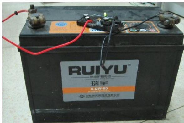
Figure 7. The battery online automatic maintenance device in the work
