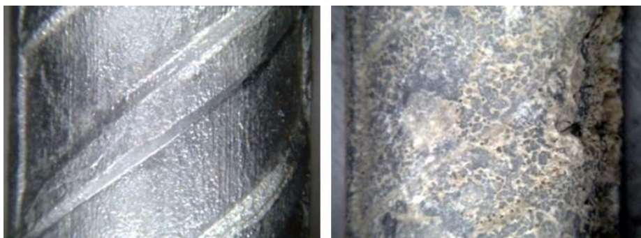
Figure 8. Surface appearance of the galvanized steel at the beginning of the experiment and after 49 days.
