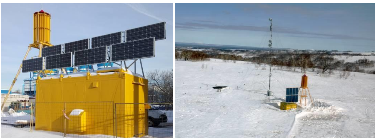
Figure 2. Hybrid power plant on the test-site (left) and in the working area (right).
